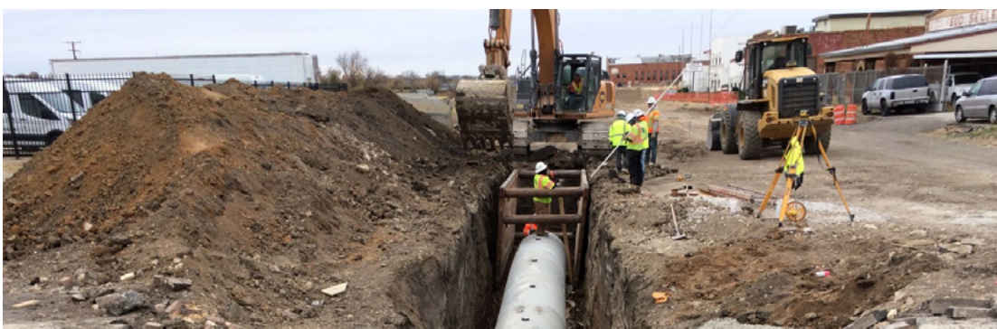
Construction still moving forward: Storm sewer being constructed north from the new manhole at NE 7th and Main Streets.
