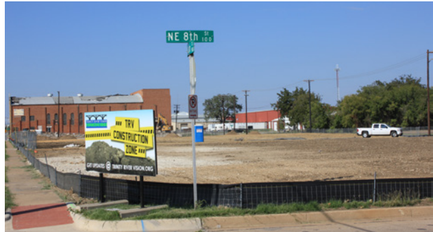
Demolition work performed by Midwest Wrecking Company of Texas, Inc.; A&R Rent A Fence; Brock Environmental Services, LLC; C. Greenscaping, LP; JD Trucking; Melgar's Transport; and Ponce Contractors, Inc.
