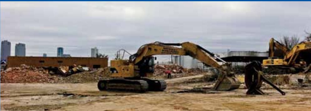
Midwest Wrecking a local Tarrant County firm, working on a demolition project at N. Main Street - clearing the way for the Bypass Channel.
